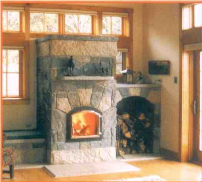
Masonry Heater with Temp-Cast precast modular core Built by Erik Nilsen, Thermal Mass Inc.
