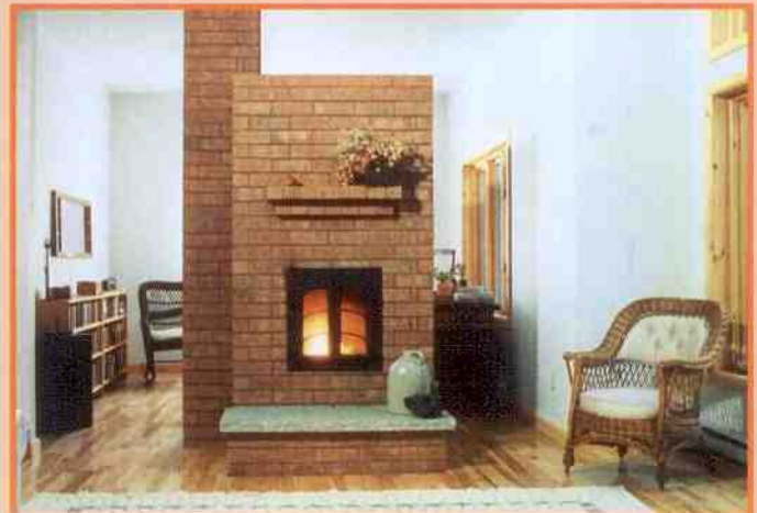
Heat-Kit Designed and Built by Norbert Senf, Certified Heater Mason Masonry Stove Builders
